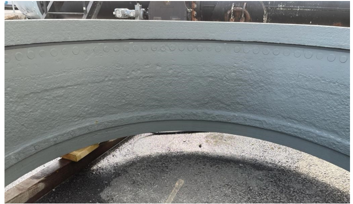
Image 2: Ex-Service expansion joint with notable severe corrosion
