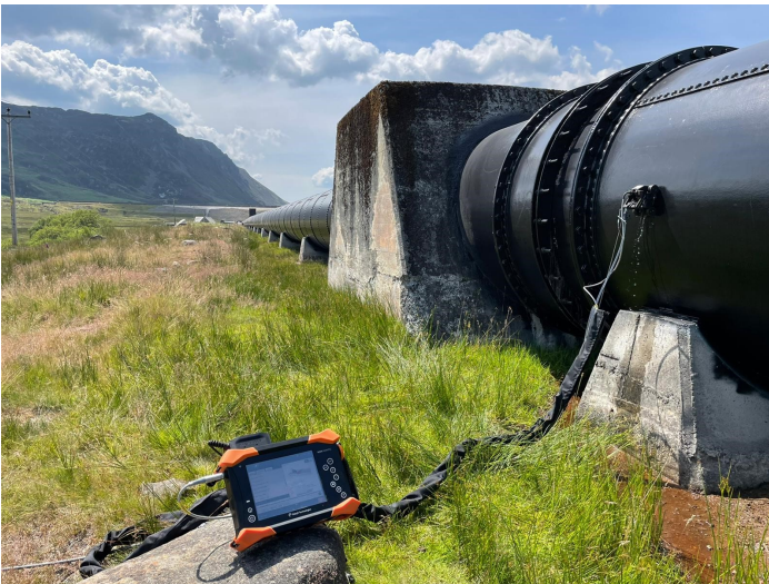
Image 1: In-situ expansion joint to the left of the R-Scan Array buggy; portable Mantis PAUT instrument also shown
