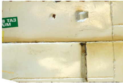
Corroded plate underside
