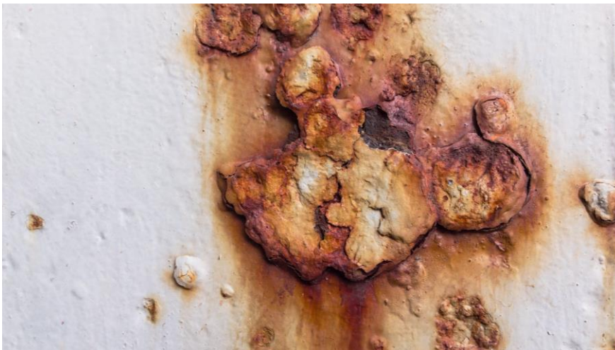
Figure 2. Corrosion scabs are typical of offshore piping systems
